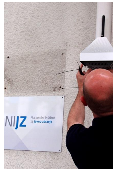
Figure 17 - Installing AQMesh at local stakeholders
